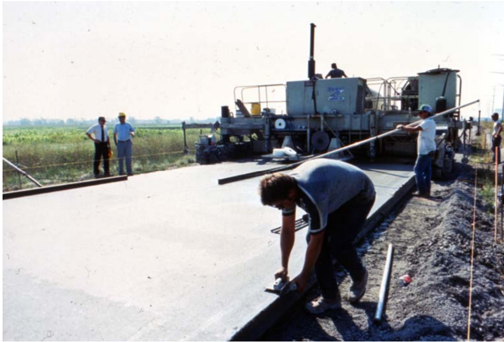
Figure 4-22: Finishing touch to We Energies' high-volume fly ash concrete demonstration project at Pleasant Prairie Power Plant..
