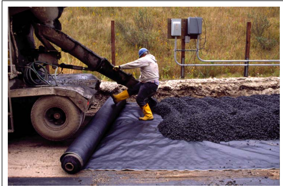
Figure 4-26: Open-graded cementitious base course material being placed over filter fabric at Port Washington Power Plant's high-volume fly ash demonstration project.
