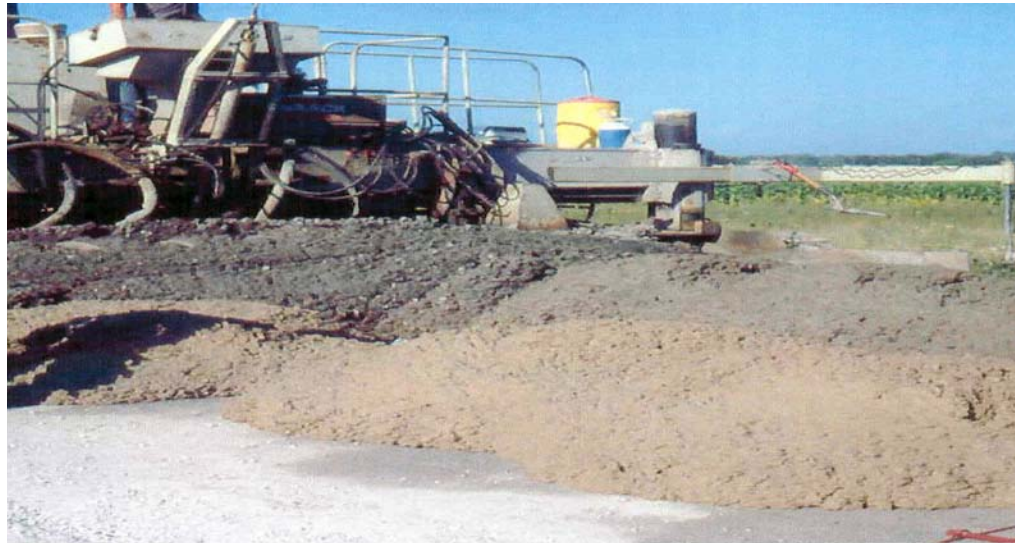
Figure 4-23: High-volume fly ash demonstration road paving at Pleasant Prairie Power Plant. Note the difference between the darker slate colored class F fly ash concrete and lighter tan colored high-volume class C fly ash concrete.
