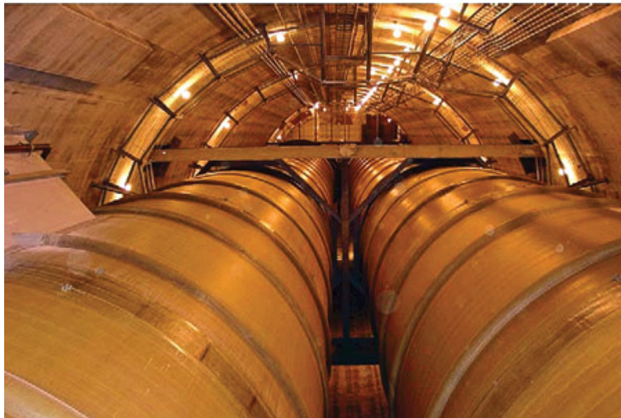
7. Two in one. The interior of the new, 430-ft tall stack, showing the two fiberglass-reinforced plastic flues, one for each generating unit. Courtesy: Washington Group International
