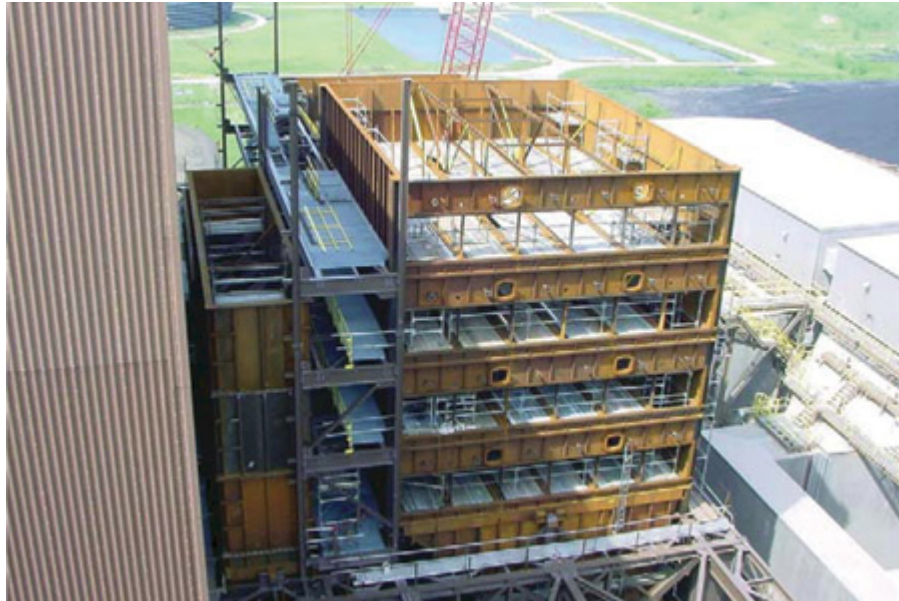
2. Clearing the air. The SCR system for Unit 1 under construction. The hot-side system is designed to remove 90% of \text{NO}_x emissions, using aqueous ammonia injection. Courtesy: Washington Group International
