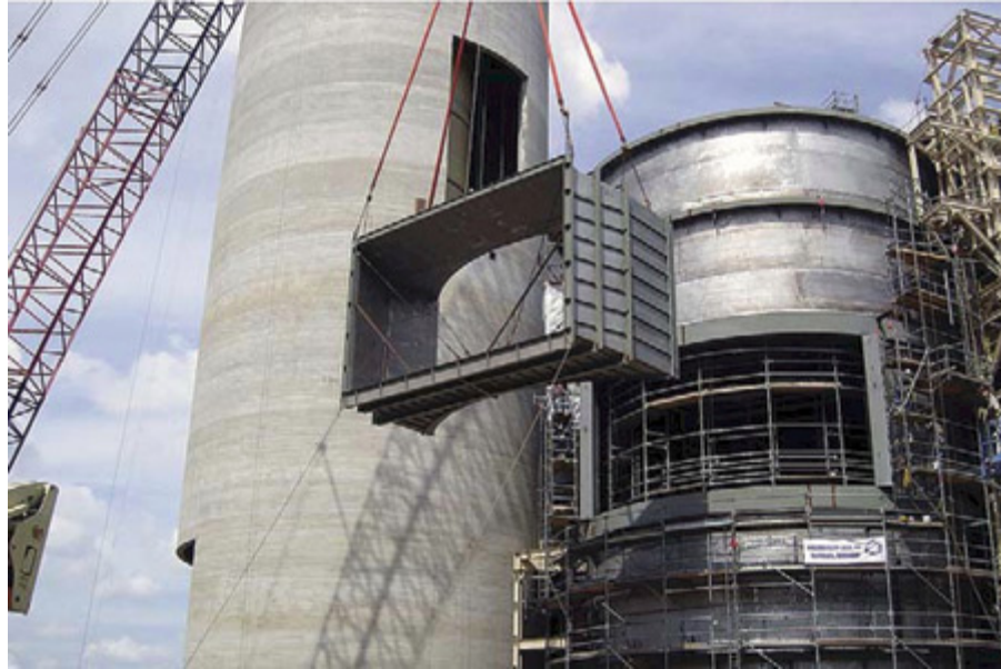
3. Scrubbing it down. The inlet to the absorber section of the new scrubber for Unit 1, shown during installation. The system is designed to remove 95% of the unit's SO 2 emissions when it's burning coal with a sulfur content of 0.5%. Courtesy: Washington Group International
