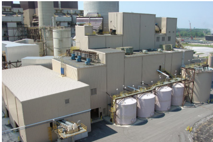
4. Compact "Scrubber Island." FGD process equipment, limestone preparation, and gypsum dewatering and storage equipment for both units are all housed in a compact design. Courtesy: Washington Group International
